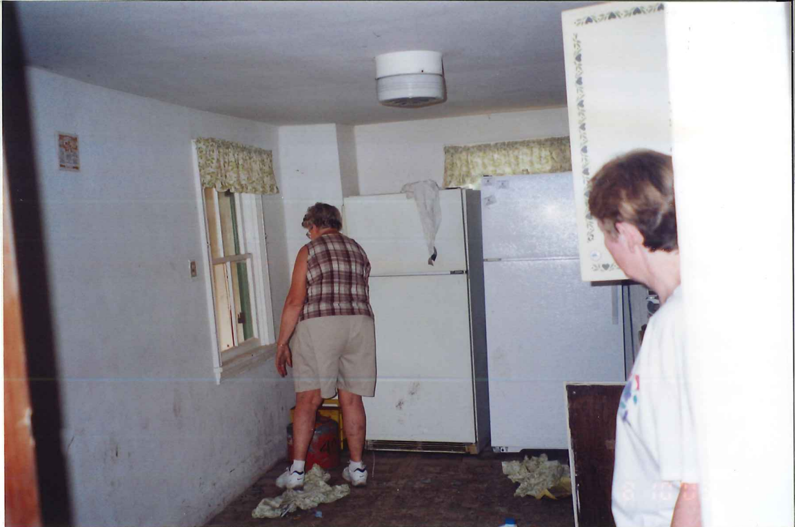
Crumbling wall & foundation of building back of house.
