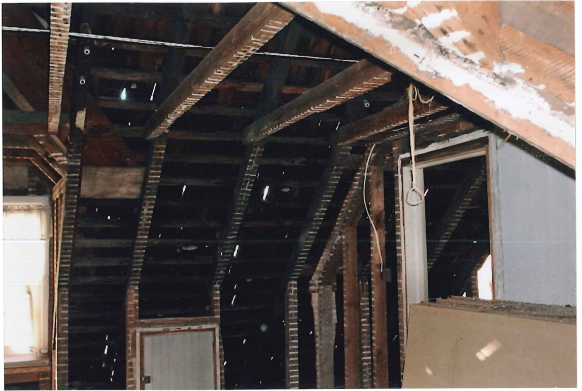
ATTIC - ROOF - SHAKES - LEAKS BADLY - CAUSING MOLD STRONG FRAMING - OLD PLASTER AND LATHE REMOVED
