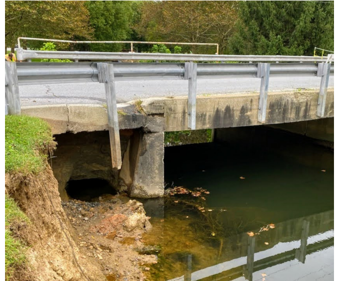
Damaged bridge at Municipal Dr. and G.O. Carlson Blvd.
