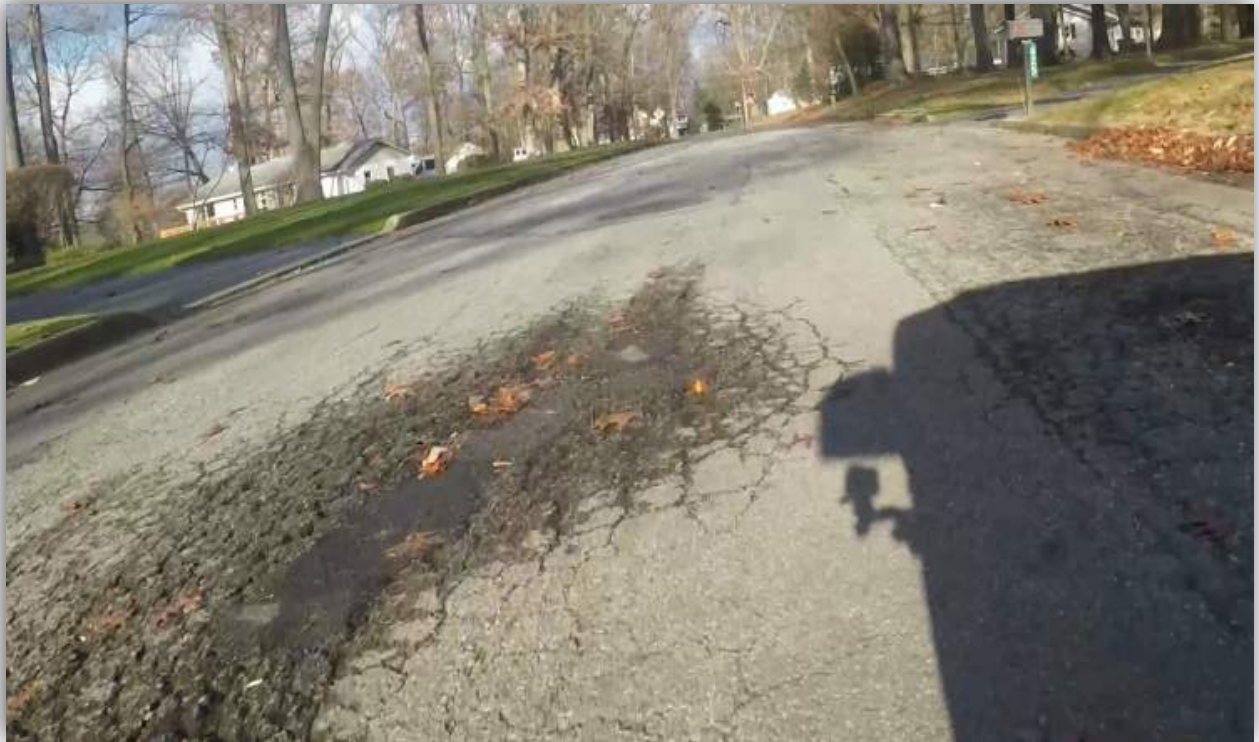
Dogwood Lane – Alligator Cracking, 5 Score
