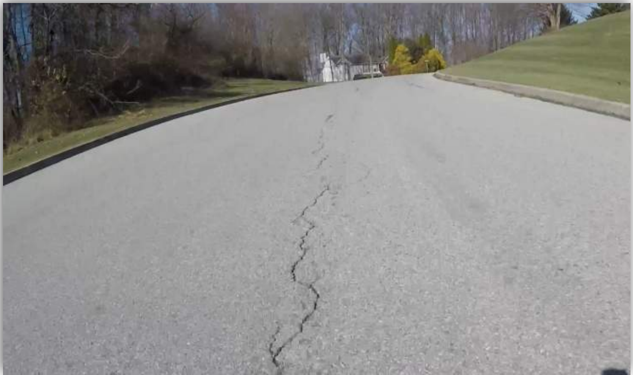
Kingswood Lane – Longitudinal Cracking, 8 Score
