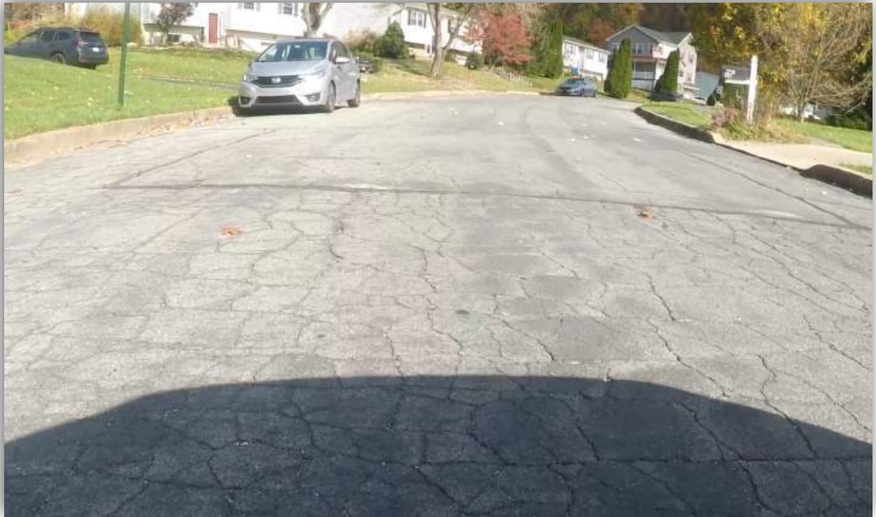
Hillcrest Drive – Block Cracking, 6 Score
