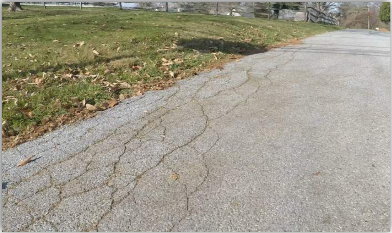
Grandview Road – Edge Cracking, 7 Score
