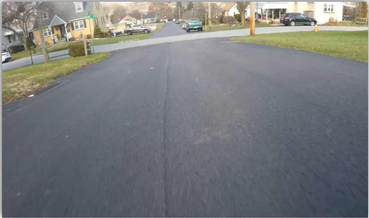
Sixteenth Street – Crack down the Centerline, 9 Score
