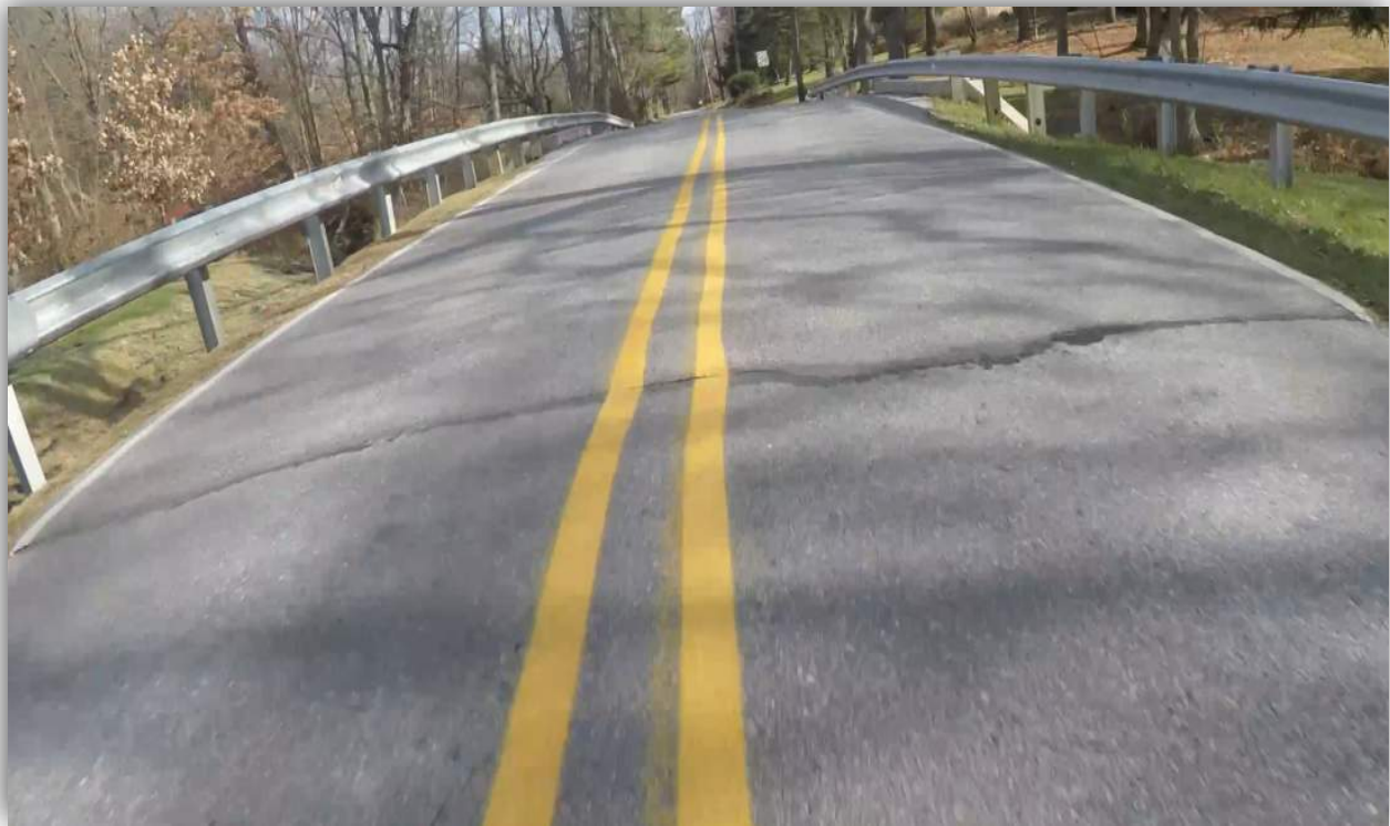
Fisherville Road – Transverse Crack, 6 Score
