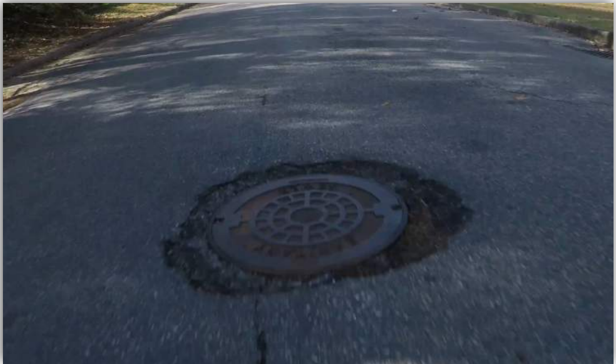
Greenwood Circle – Pothole around Manhole, 7 Score
