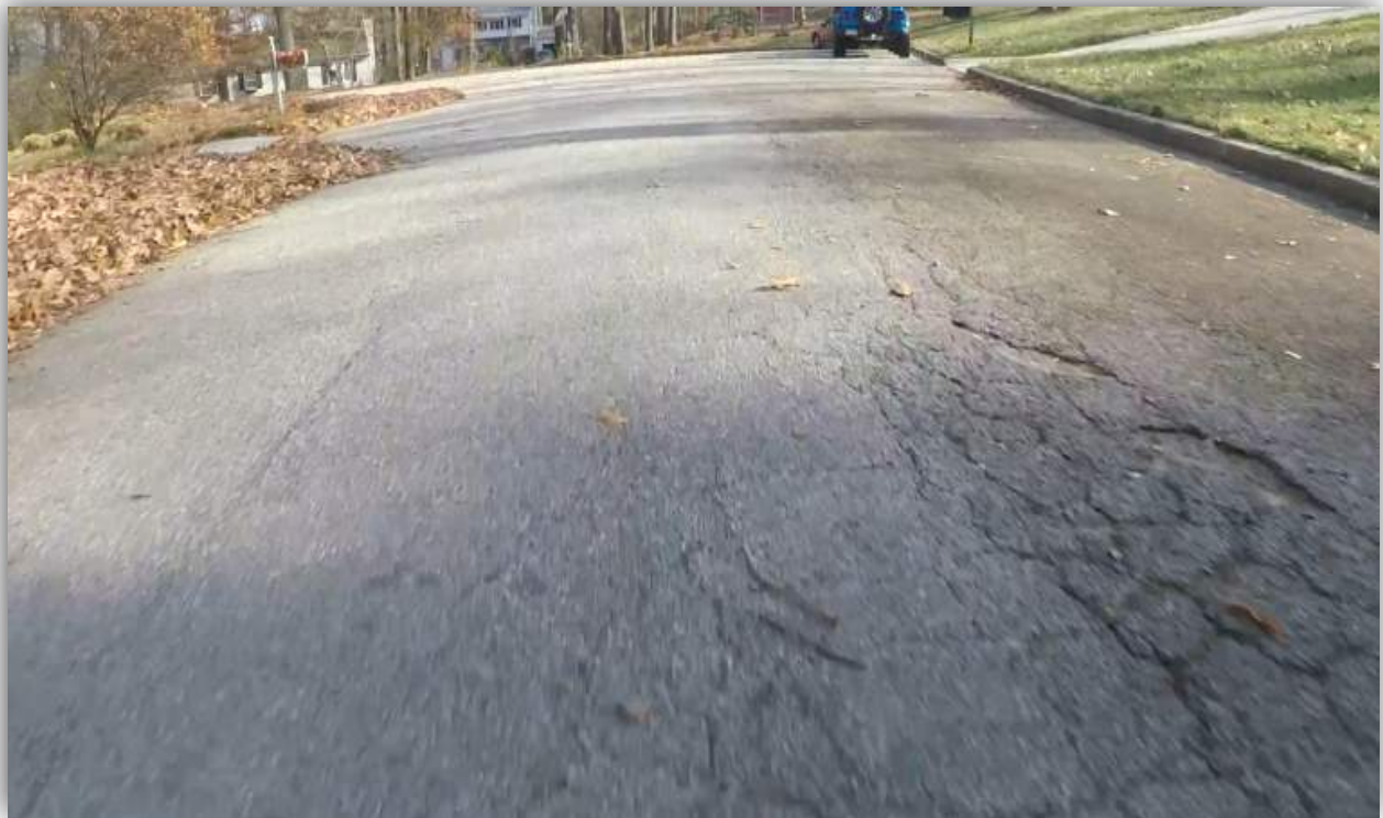
Woodview Drive – Alligator Cracking & Raveling, 7 Score
