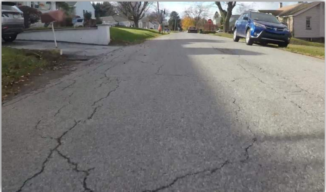
Norwood Avenue – Cracking, 6 Score
