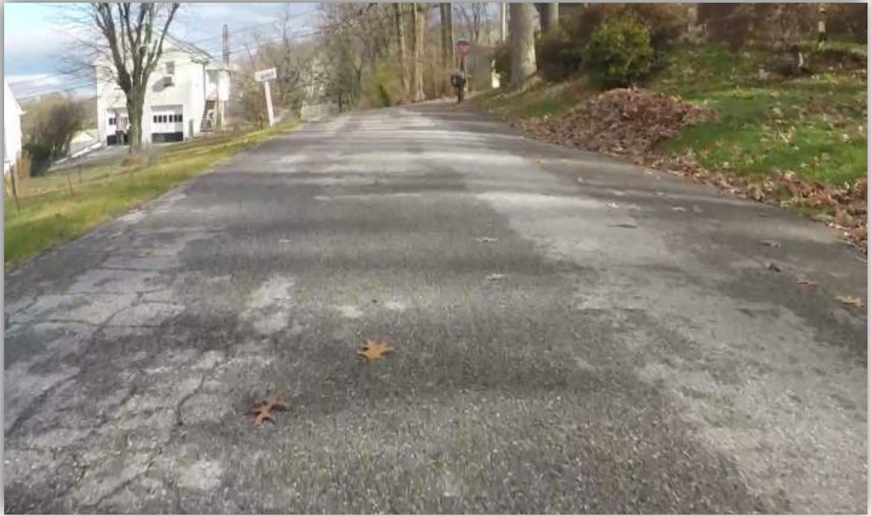
Bungalow Glade – Block Cracking, 6 Score
