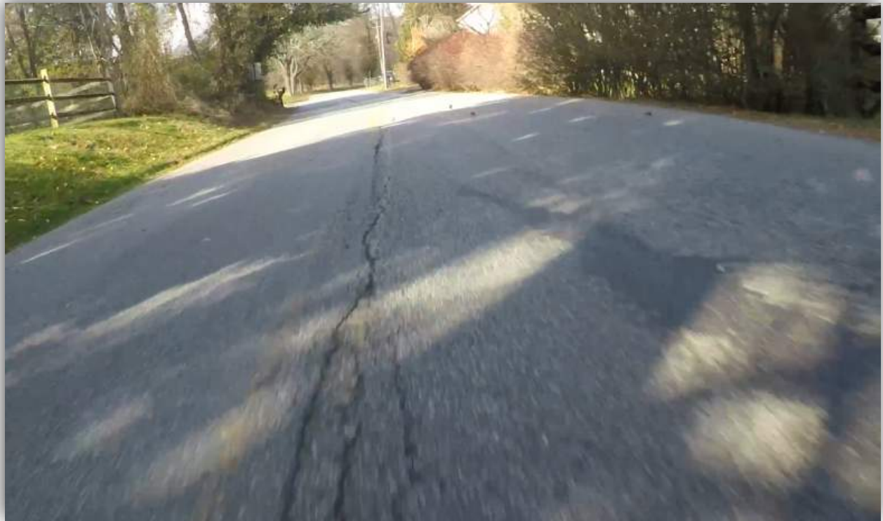
South Caln Road – Longitudinal Cracking along Centerline, 7 Score
