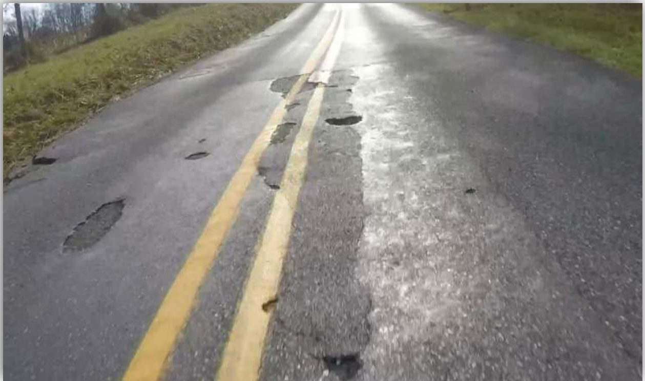
North Bailey Road (North) – Potholes & Raveling, 6 Score
