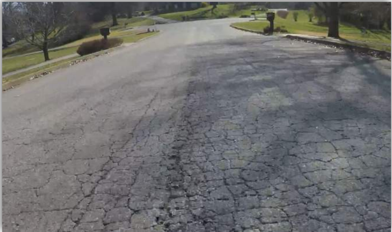
Schoolhouse Lane – Alligator Cracking in Small Area, 7 Score
