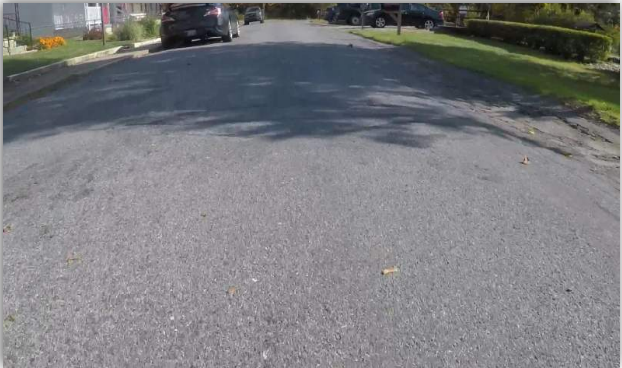
Maple Avenue – Depression & Raveling, 6 Score
