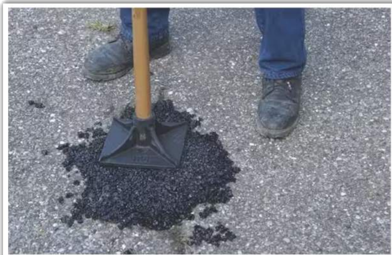
Figure 1: Cold Patch Repair
