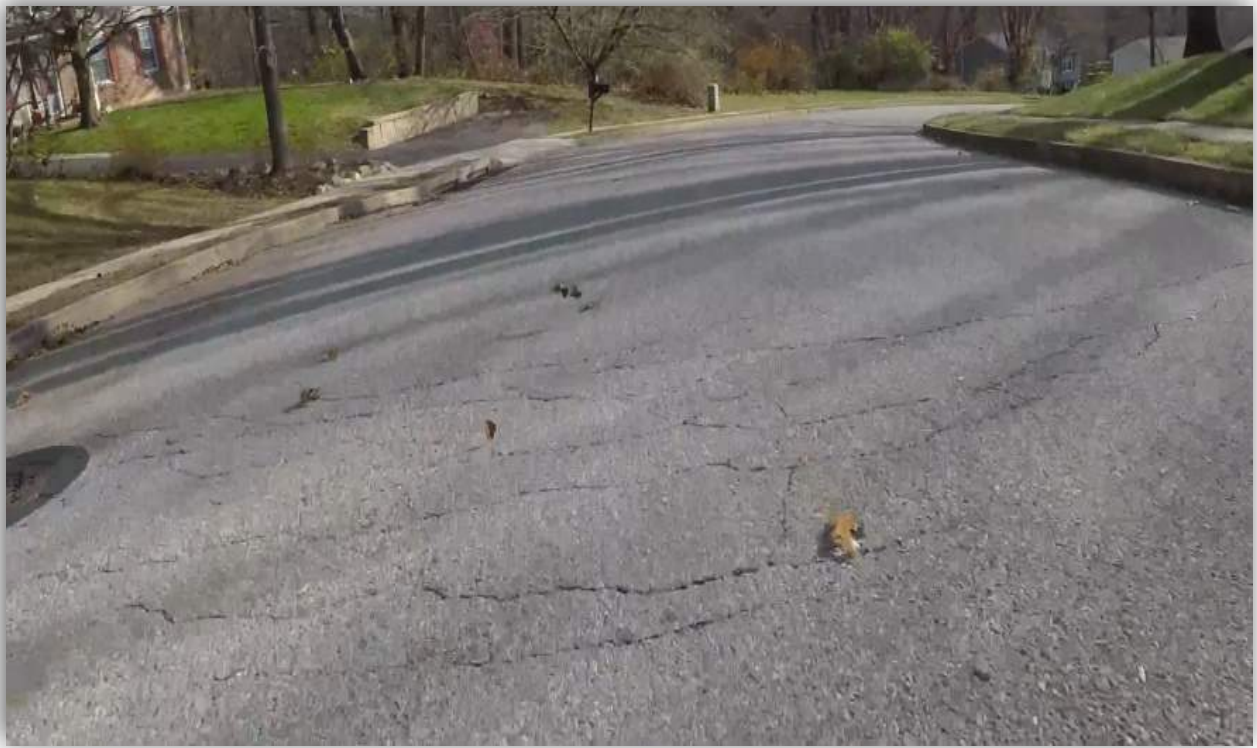
Jennifer Drive – Transverse Cracking, 7 Score
