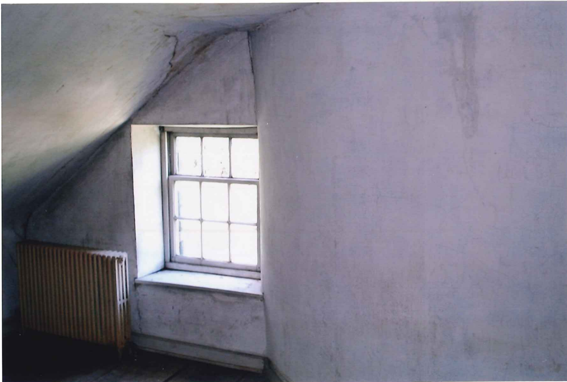
ATTIC FACING EAST REAR ROOM - WHAT IS LARGE ROUNDED WALL OBJECT?
