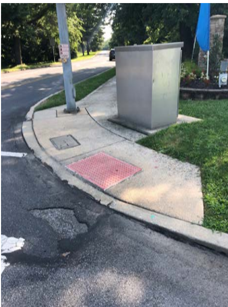
Above: The pedestrian curb ramp at the intersection of G.O. Carlson Boulevard and Bondsville Road.
